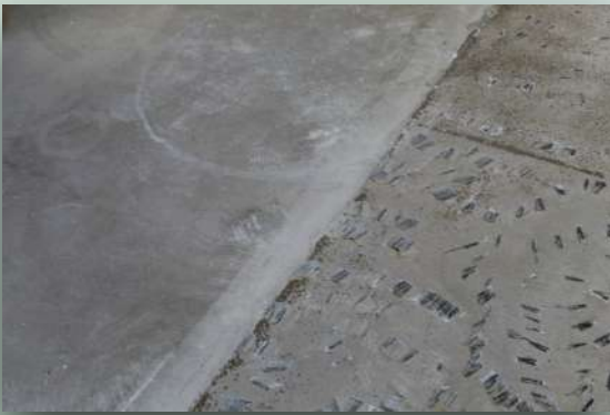
Here you can see a relatively good underfloor (on the left) and one that needs some treatment (on the right).
